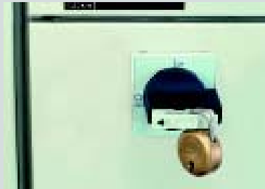
Door interlocks & padlocking facility.
