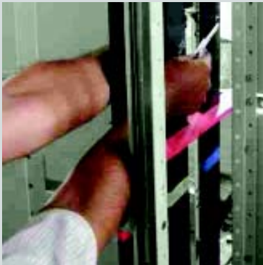
Access to the last vertical busbar available from both sides.
