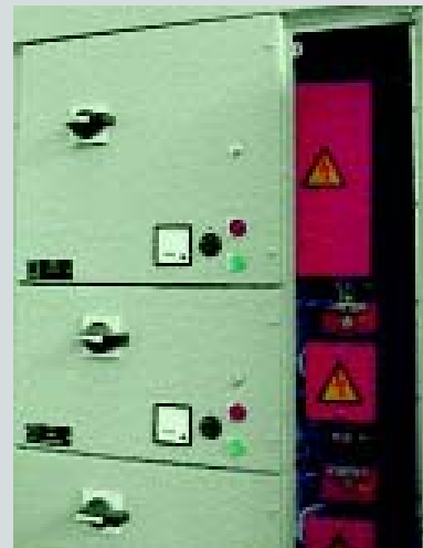
Totally shrouded Power terminals.
