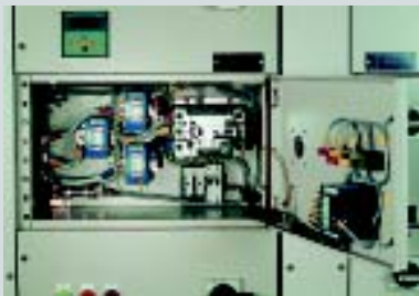
Module width of 500 mm facilitates safe & easy equipment replacement.
