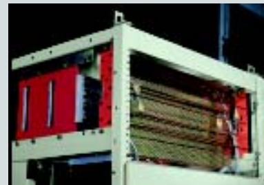
Main busbars and control busbars are totally segregated from each other. Upto 11 number control bus per panel.
